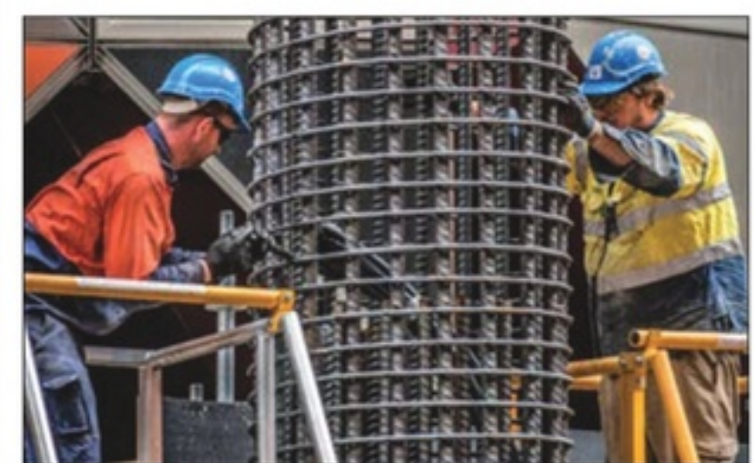
Figure 2- a) Thermally activated retaining wall b) Geothermal pipe installation (State Government of Victoria, 2024).
