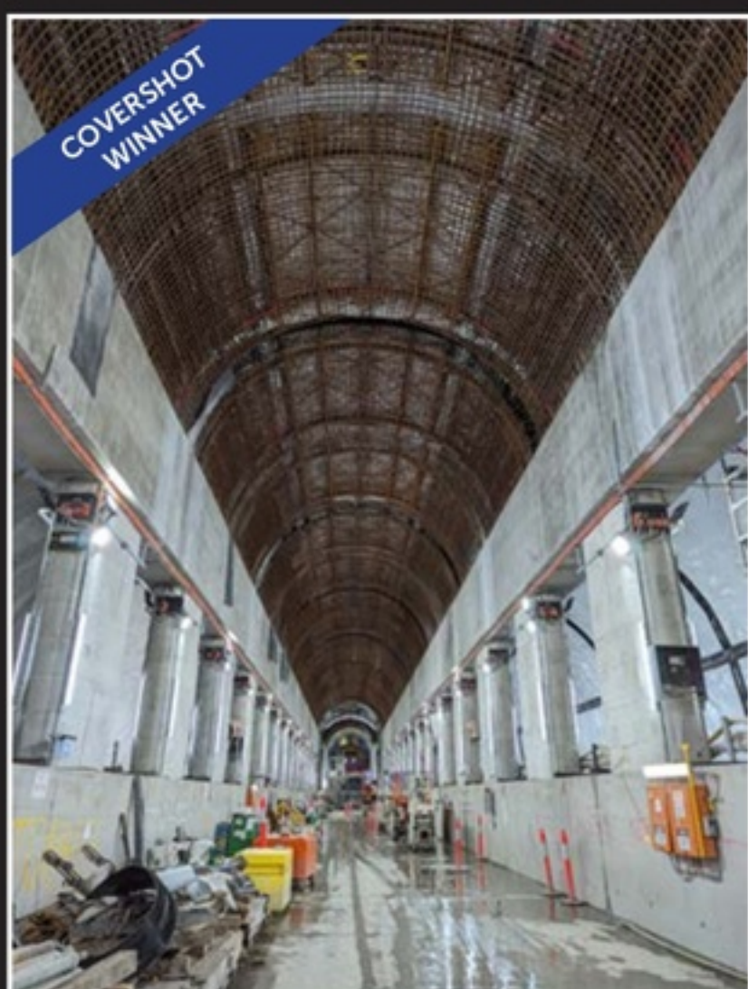
An assembly of self-supporting prefabricated arch reinforcement cage in the Town Hall Station cavern beneath Swanston Street. Melbourne Metro Tunnel Project, by Vern Lee
