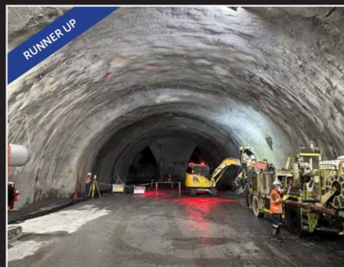
Infill spraying process - Sprayed shotcrete process creating tunnel profile arch. Brisbane Metro Acciona ARUP JV, by Dallas Adams
