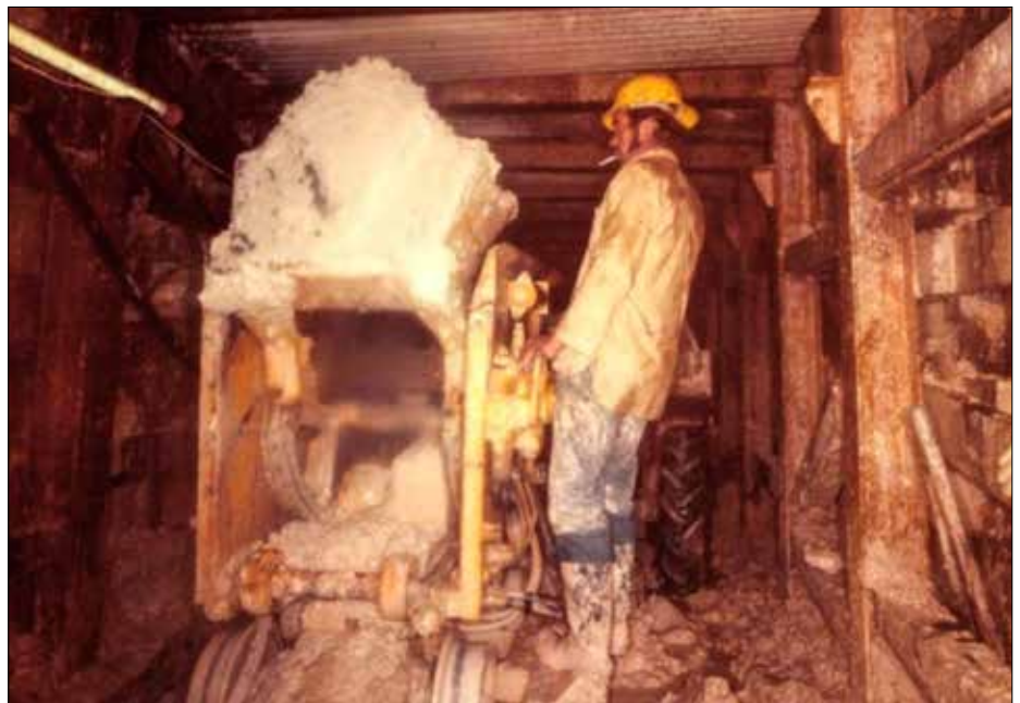
Digging the pilot tunnel for the Melbourne Underground Rail Loop (MURL) in August 1972. MURL was another of the reasons that tunnelling in Australia was seen as an industry in need of its own agency. Note the cigarette – a sign of how much society (and underground safety, has changed since the 70s. Photo: Public Record Office Victoria
