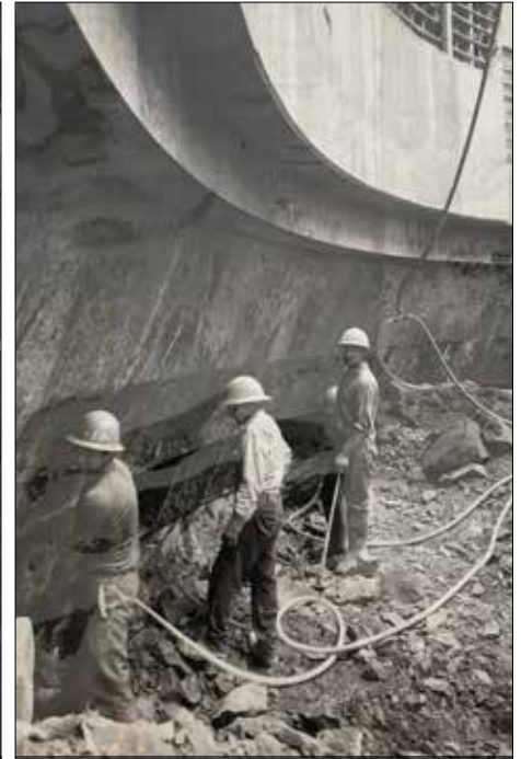
The sinking of the caisson onto a sloping rock face for the North Road Pumping Station.
