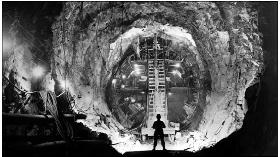
The Snowy Hydro Scheme was one of the reasons that tunnelling in Australia was seen as an industry in need of its own agency.
