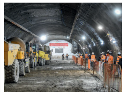
The Town Hall site of the Metro Tunnel, which was connected to the Federation Square site in June 2020, was shut down after two workers tested positive to COVID-19.
