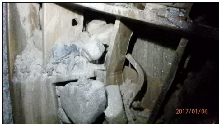
Figure 14: Damaged and bent grizzly bars allowing boulders larger than 250mm to enter the excavation chamber
