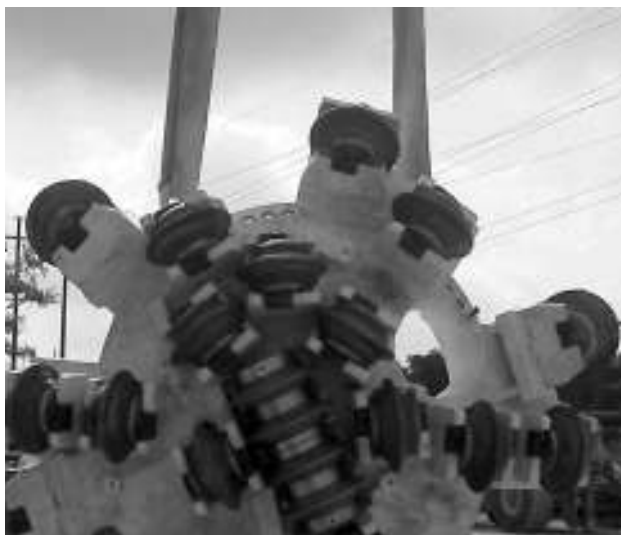
The cutterhead lowering of a high-powered Robbins Main Beam TBM boring the Jollyville Transmission Main in Texas, USA.
