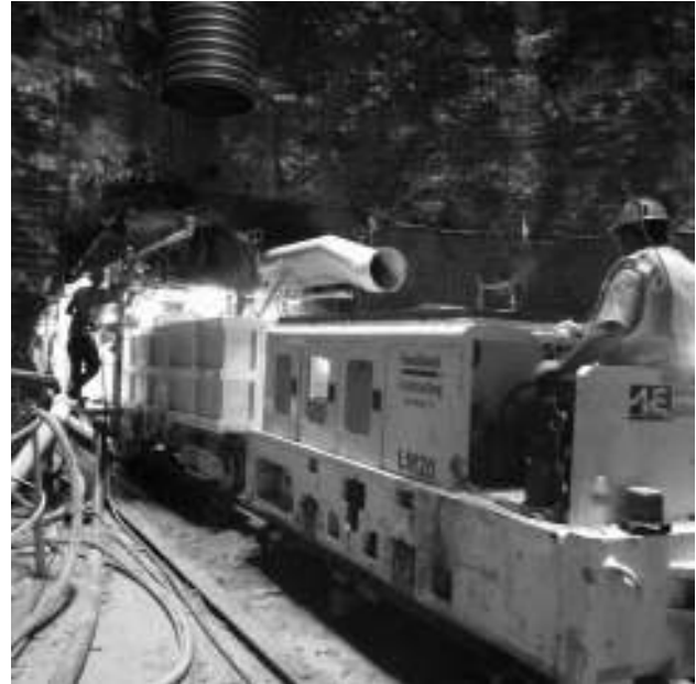
The smaller size of the 3.25 metre (10.7 feet) Robbins Main Beam tunnel requires thorough logistical planning by the Southland/Mole JV.
