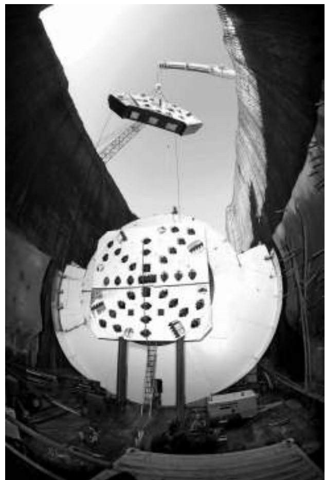
Robbins developed its highly successful Onsite First Time Assembly (OFTA) method for the Niagara Tunnel Project in 2006.
