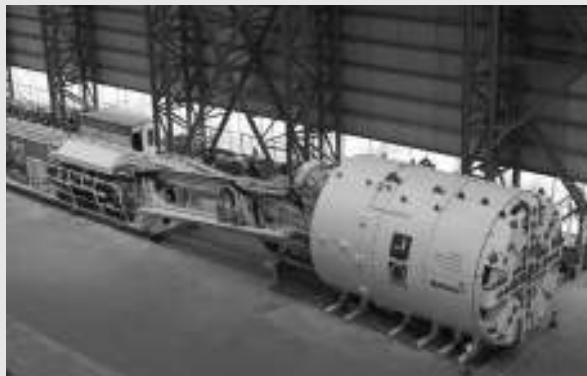
Russian contractor Engeocom is using three EPBs, including two new Robbins machines between Business Center and Park Pobedy Stations.
