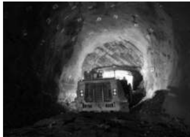
The underground block-cave project is large and complex, requiring more than 40 kilometres of tunnelling.
