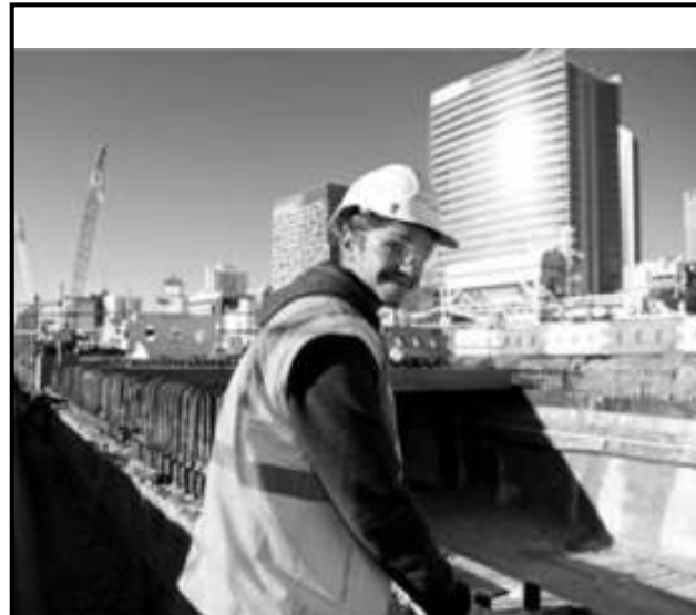
Trainee Orace Hayden has found the Fremantle tunnel project offers more challenges than his last job.
