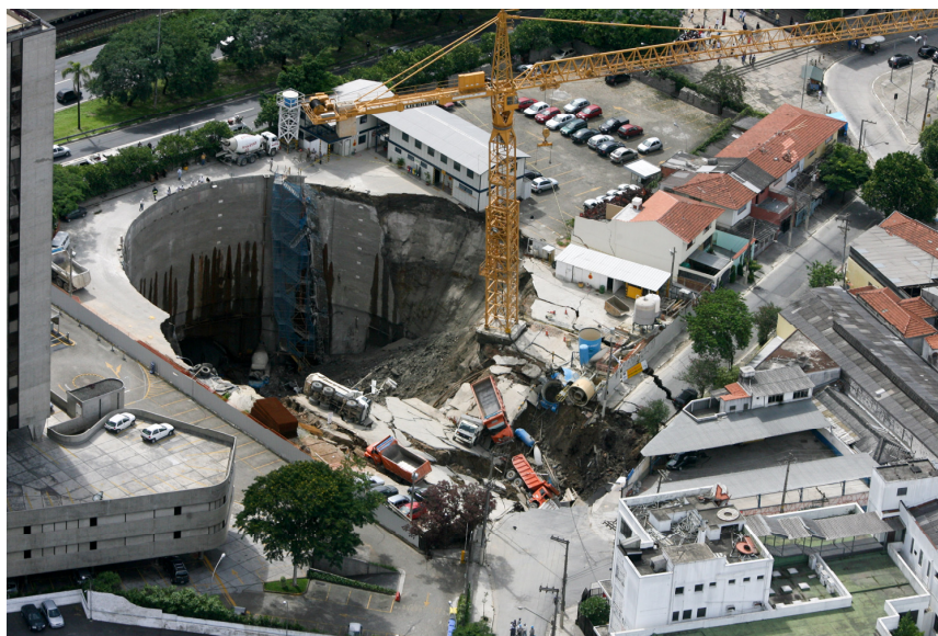
Fig. 2. São Paulo Metro station collapse (photo courtesy of Ayrton Vignola/ Folha de S.Paulo).
